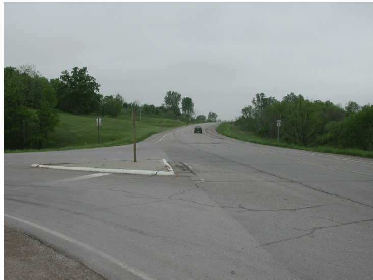
Looking south on Ia. 5 from T30 at limited sight distance and horizontal curvature.
